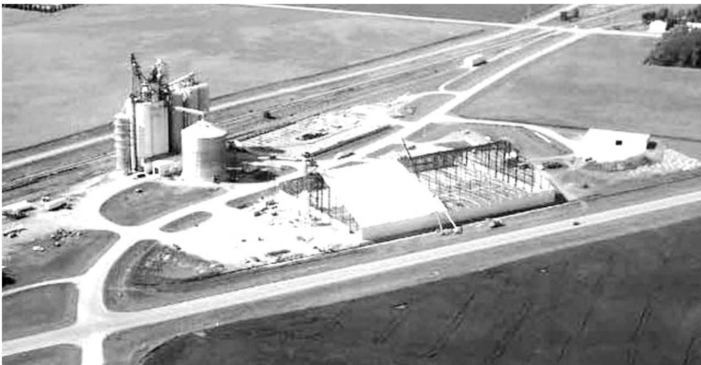
David Oftedahl was being piloted by Jon Wolff over Hanley Falls last month when he snapped this photo of our new Grain Storage Shed being constructed, south of the main office. The 300-foot wide, 450-foot long unit will hold approximately four million bushels of corn and will be completed by harvest. We'll be hosting an Open House Thursday, Sept. 13, and serving pancakes and sausage from 4 to 7 p.m.
